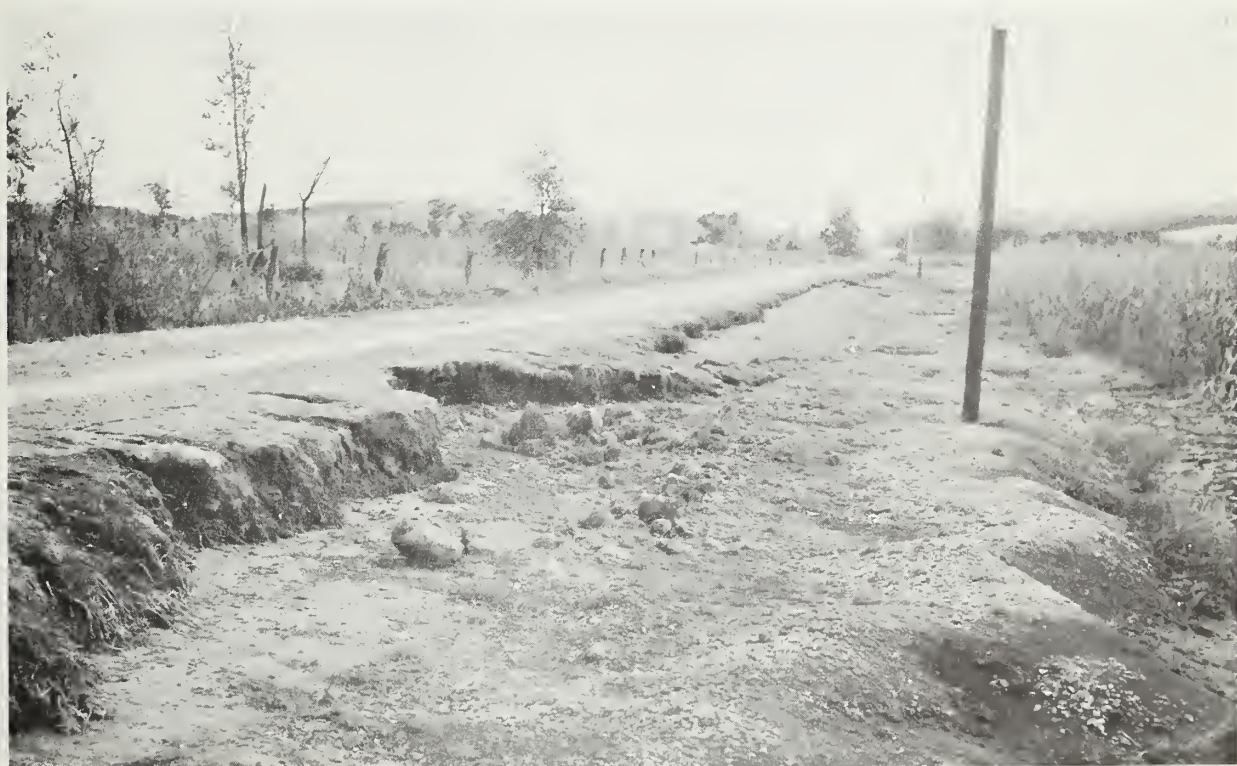
Flood flows caused erosion damages to this road bed.
